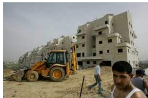
Arab workers construct new housing units for Jewish settlers in the West Bank settlement of Givat Zeev in March of this year. AP
